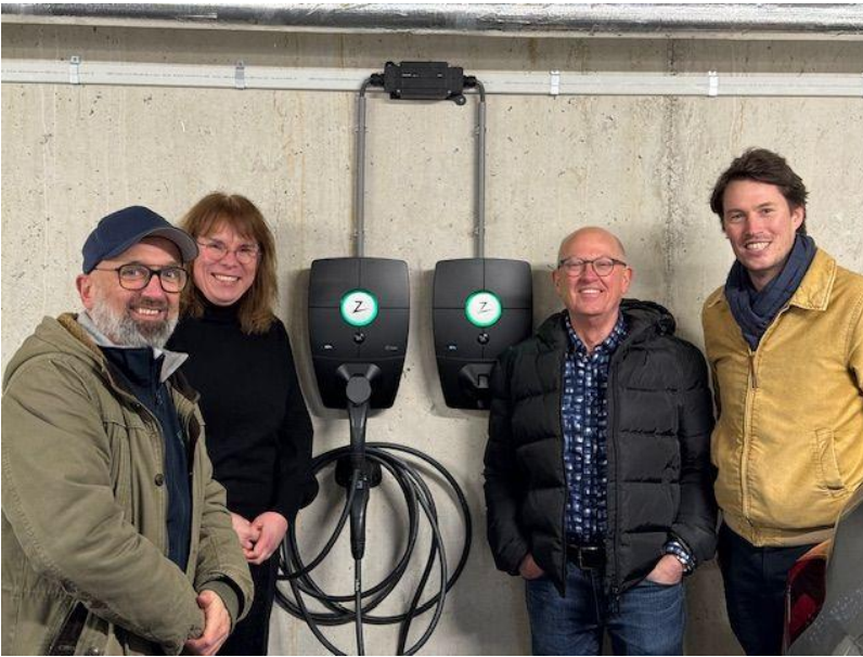
Fig 7: installation of two shared charging points in Purmerend apartment building
